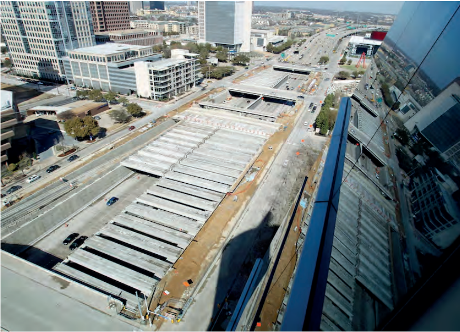
Concrete box beams being laid over Woodall Rodgers Freeway to support the deck of Klyde Warren Park in 2011. (File photo / 2011) (Vernon Bryant/Staff Photographer / dallas morning news)
